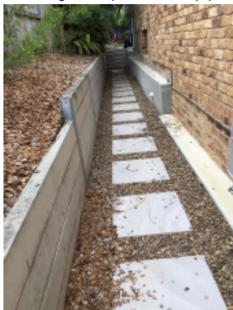
Showing example of areas with poor drainage
