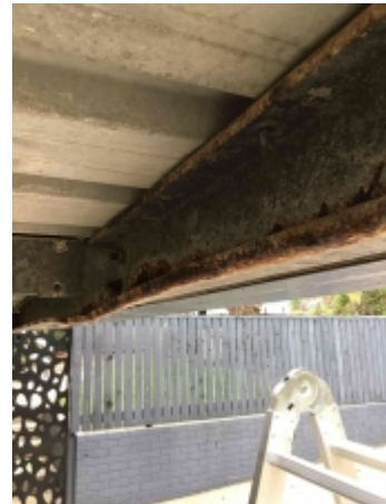
Rusting to parts of carport framing, recommend a builder to repair or replace and avoid further deterioration
