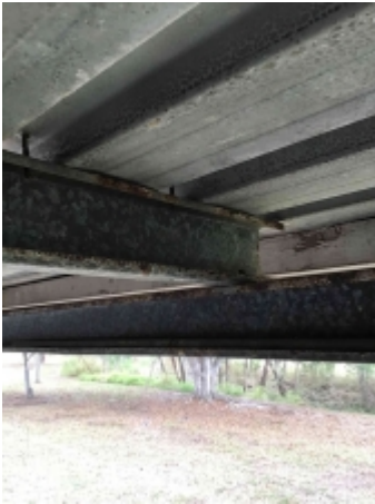
Rusting to parts of carport framing, recommend a builder to repair or replace and avoid further deterioration
