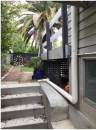
Showing example of insufficient balustrading
