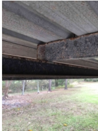
Rusting to parts of carport framing, recommend a builder to repair or replace and avoid further deterioration
