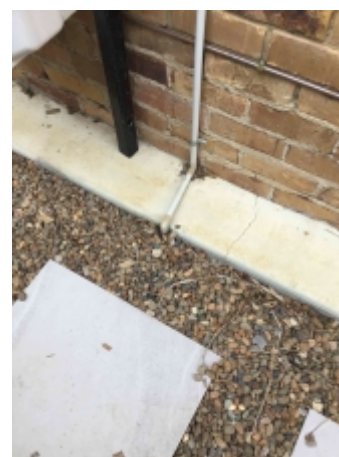
Showing example of AC unit overflow
