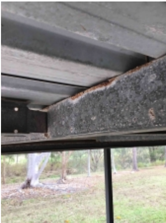
Rusting to parts of carport framing, recommend a builder to repair or replace and avoid further deterioration
