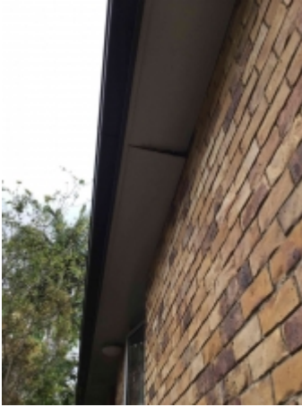
Showing loose soffit sheets
