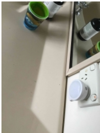
Cracked/loose/missing sealant/grout to parts of bathroom. Recommend resealing to reduce the risk of water leaks and damage
