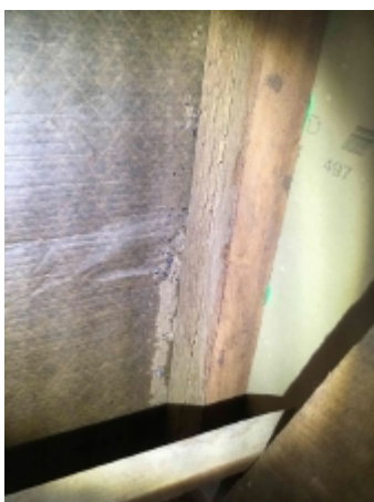
Termite damage to parts of the roof framing. Recommend engaging a builder for further invasive inspection to the area to determine if there is any concealed damage and replace all damaged timbers., Lower level roof space
