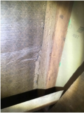
Showing example of termite damage
