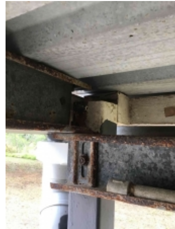
Rusting to parts of carport framing, recommend a builder to repair or replace and avoid further deterioration
