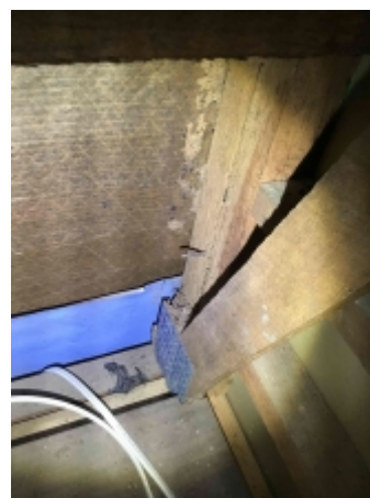
Termite damage to parts of the roof framing. Recommend engaging a builder for further invasive inspection to the area to determine if there is any concealed damage and replace all damaged timbers., Lower level roof space
