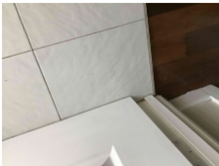
Cracked/loose/missing sealant/grout to parts of bathroom. Recommend resealing to reduce the risk of water leaks and damage
