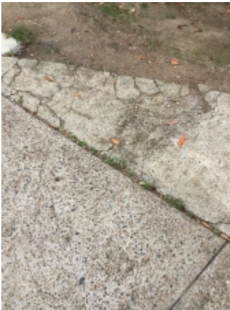
Settlement cracks to parts of the pathway/driveway. Recommend engaging a concreting contractor to repair/replace and avoid further deterioration
