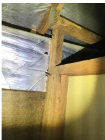
Termite damage to parts of the roof framing. Recommend engaging a builder for further invasive inspection to the area to determine if there is any concealed damage and replace all damaged timbers., Lower level roof space
