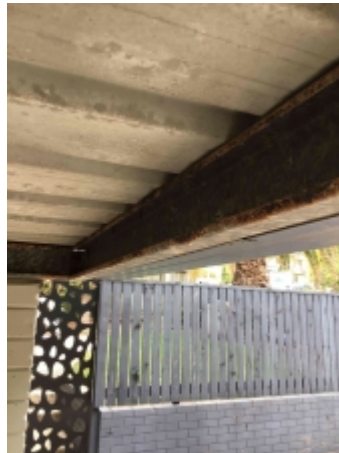
Rusting to parts of carport framing, recommend a builder to repair or replace and avoid further deterioration
