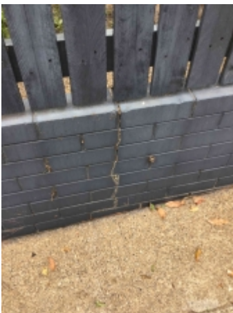
Cracked retaining wall to the front elevation, recommend a builder to repair or replace and avoid further deterioration
