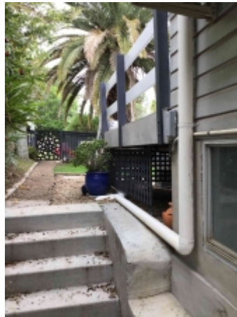
Insufficient balustrading to the external areas, balustrading should be minimum 1000 high for the patios/balconies and 865 mm for the stairs with gaps no greater than 125mm, rectify to reduce the risk of personal injury
