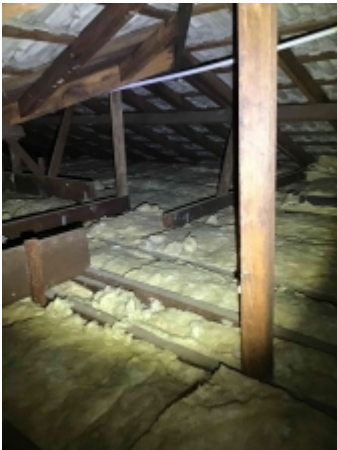
Showing examples of obstructions (e.g. wall, floor, ceiling coverings, cabinets, window furnishings, vegetation, insulation and ducted AC, furniture and stored goods, etc.)
