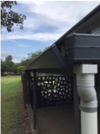
Loose flashing to the carport roof, recommend a plumber to repair or replace and avoid further deterioration
