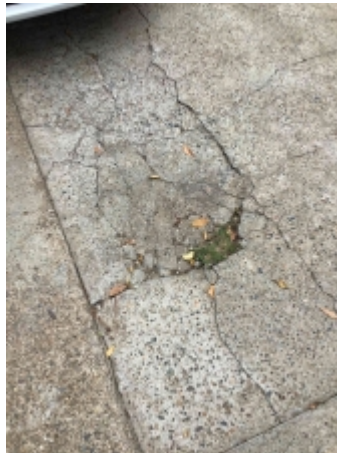
Settlement cracks to parts of the pathway/driveway. Recommend engaging a concreting contractor to repair/replace and avoid further deterioration
