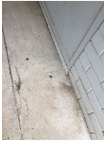
Showing example of bridging
