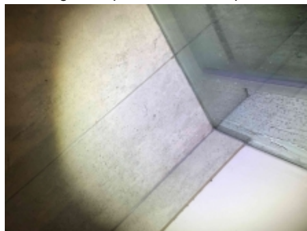
Showing example of areas with leaks
