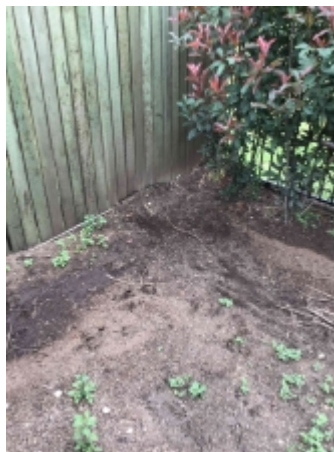
Parts of the fences are in ground contact. Recommend exposing 75mm under the timbers to reduce the risk of wood rot and termite attacks
