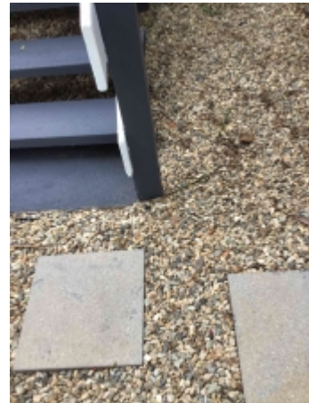
A few timbers are in contact with the ground. Recommend exposing a minimum of 75mm under all timbers to reduce the risk of termite attack and wood rot
