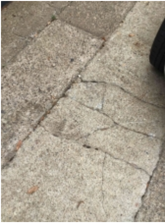
Settlement cracks to parts of the pathway/driveway. Recommend engaging a concreting contractor to repair/replace and avoid further deterioration
