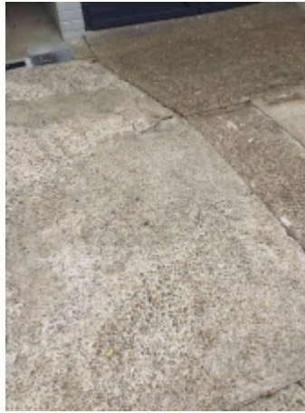
Settlement cracks to parts of the pathway/driveway. Recommend engaging a concreting contractor to repair/replace and avoid further deterioration
