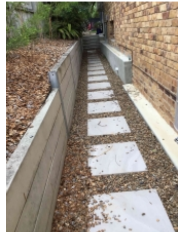
Poor surface drainage – needs improvement to reduce the risk of footing movement and other moisture related issues
